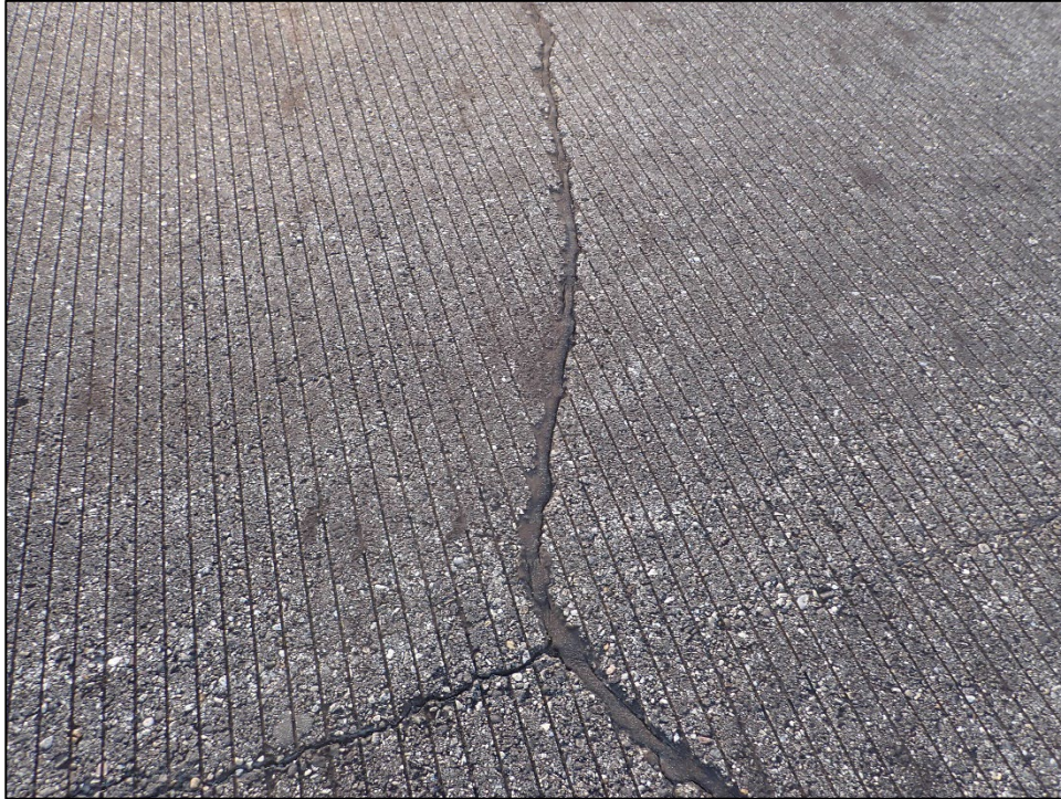
RW01-01-85: L&T Cracking
