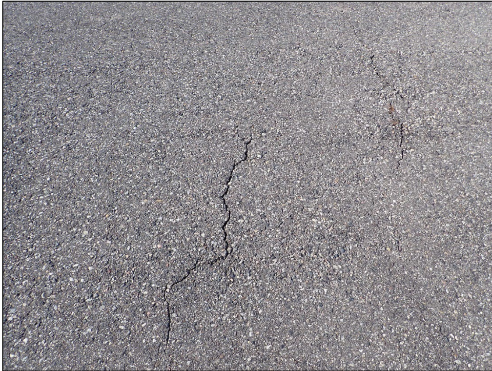
TW-02-02: L&T Cracking
