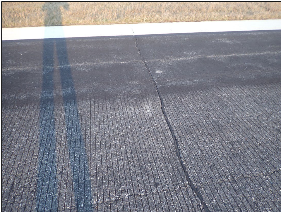
RW01-02-28: L&T Cracking
