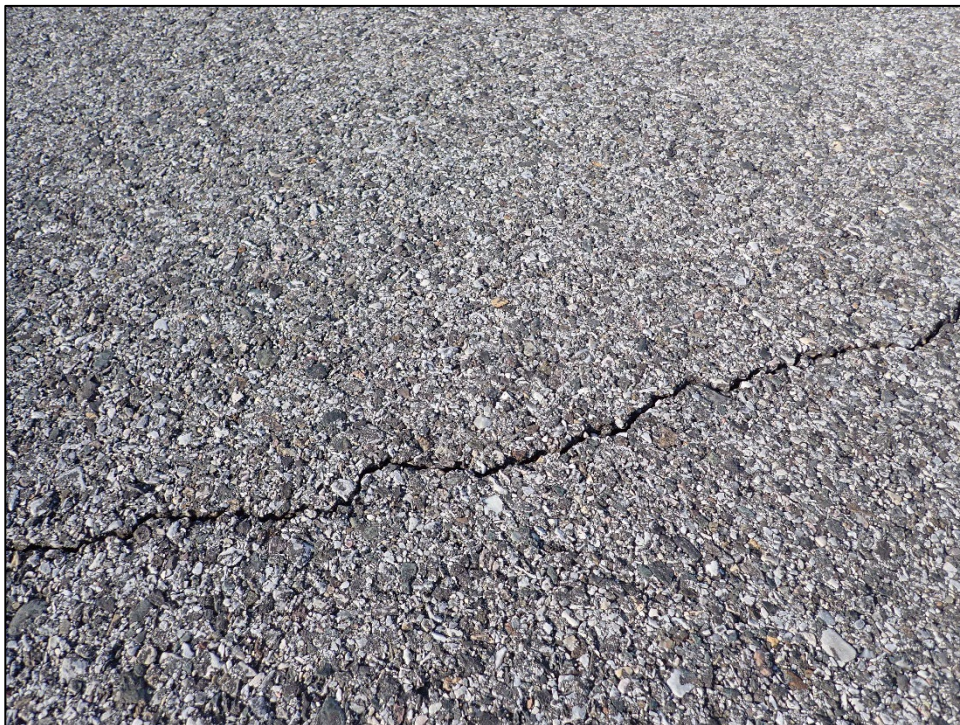
TW-11-145: L&T Cracking
